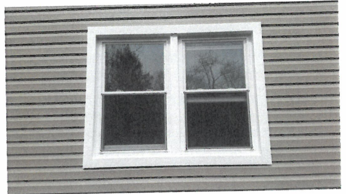
Is the trim the city requires not easily purchased?
