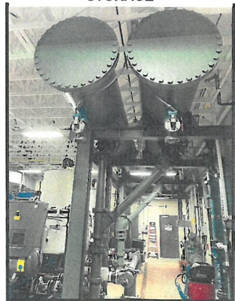
FIGURE 2-6: RAW WATER STORAGE
